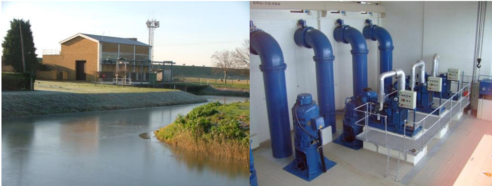
Figures 7-10 and 7-11: Cross Guns Pumping Station inside (left) and outside (right). Source: North Level District IDB
